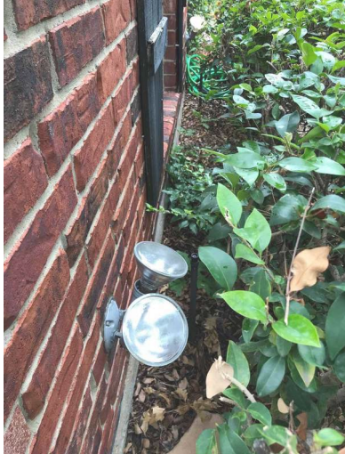
Front Yard Uplights
